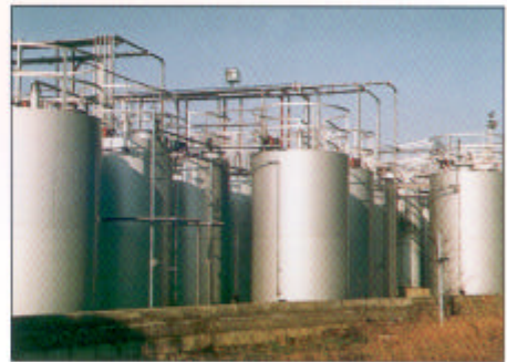
Tank farm inventory. Resins and solvents.
